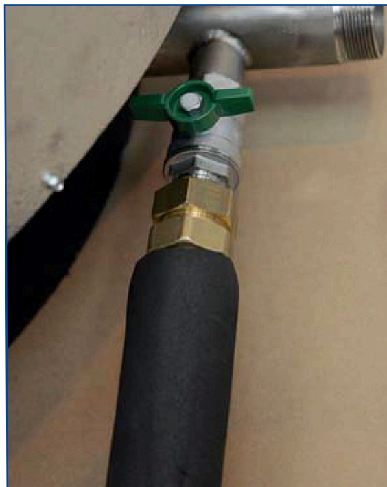
14. Insure the flexible hose connection is tight.
