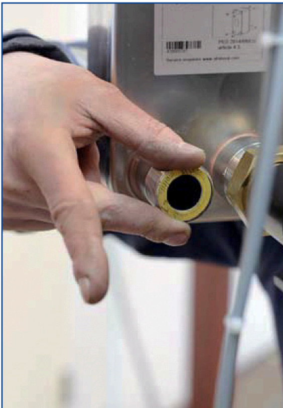
7. Install a fibre washer on the inlet connection of the heat exchanger.
